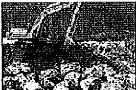
Excavation SR-2. Crews observed removal activities to verify paint waste was removed. More than 47,000 tons of paint waste and other materials was removed from the 15 SR areas and the disposal areas.
