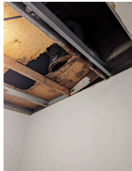
Photo 8 – Missing ceiling inside Benjamin Moore store
