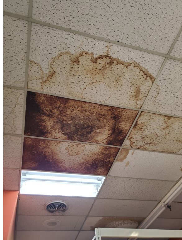
Photo 7 – Water damage inside Benjamin Moore store
