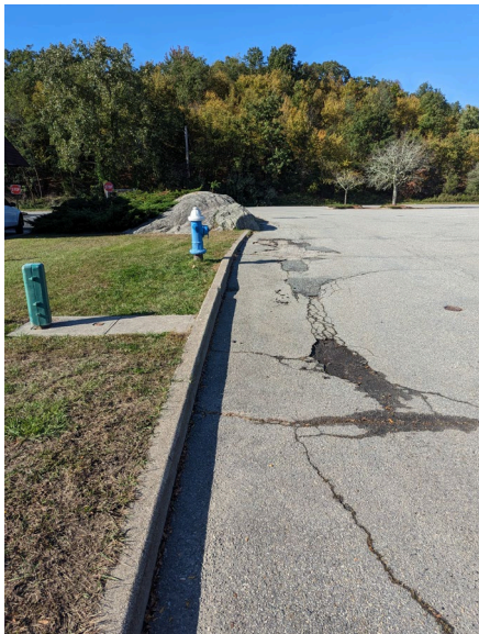
Photo 11 - Cracked parking area pavement
